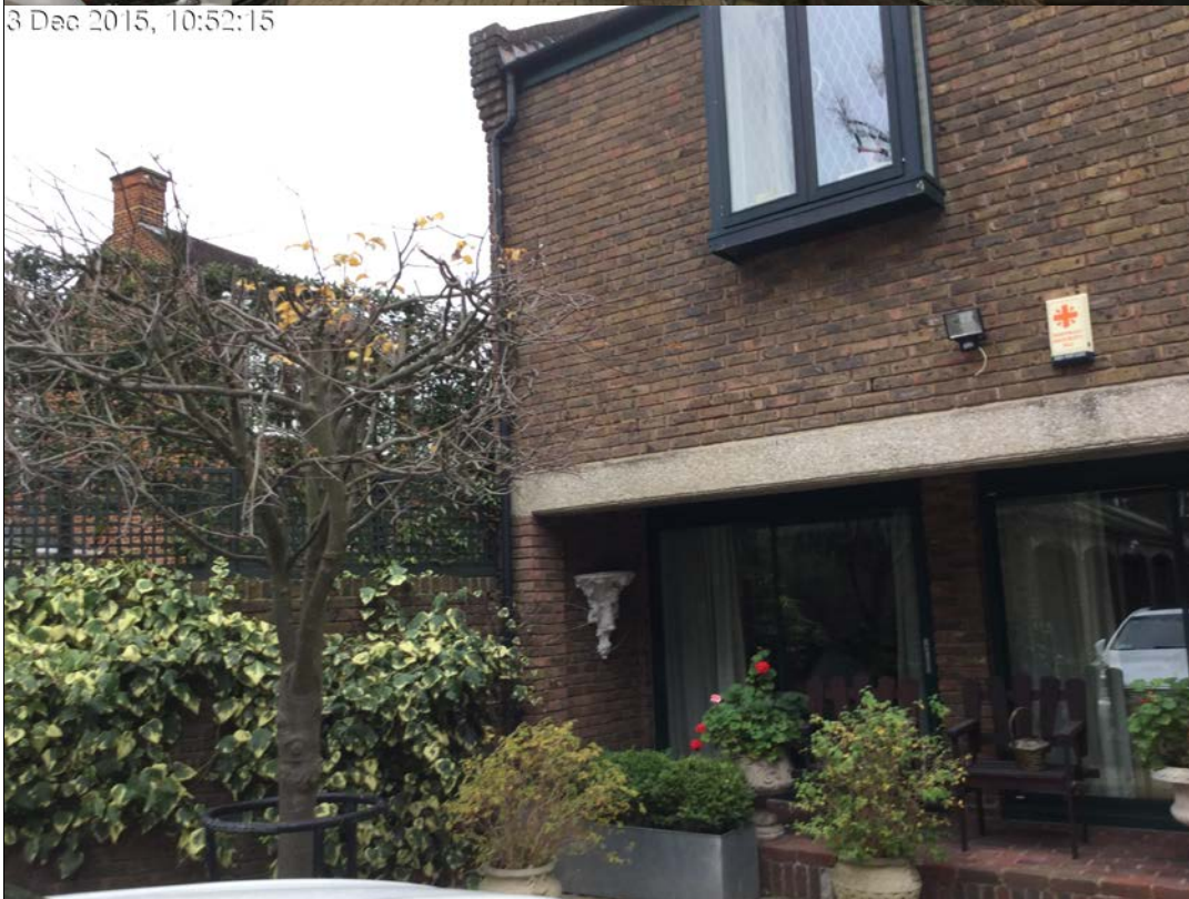
Below: View of the affected recessed window at ground floor level.
